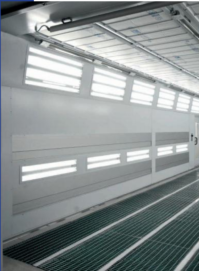
Full grids on concrete works with frames under the grids with adjustable downdraft flow.
